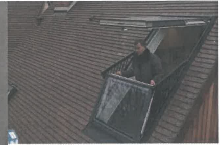
NOT PERMITTED: Roof window at irregular angle
